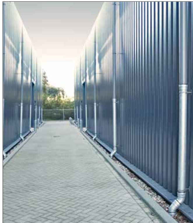
LORO-X rain standpipes without clean-out openings with pipe offset into the sewer pipe
